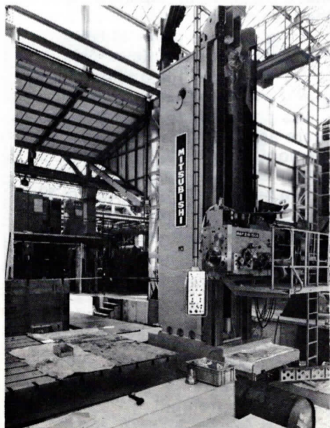
B & S Massey's new ram borer machine being installed in their heavy machining bay.
