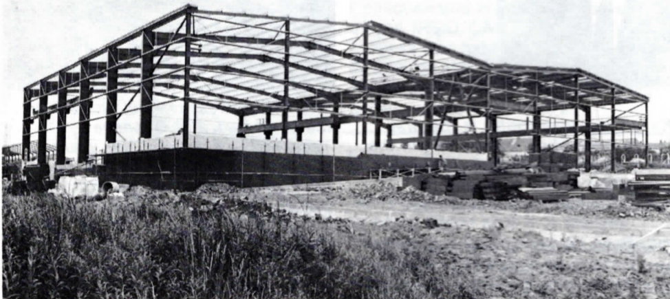
Progress photograph taken in July of the new Wrightstock warehouse at Worsley under construction. (Photo by courtesy of A Lancaster Britch & Associates, Chartered Architects).
