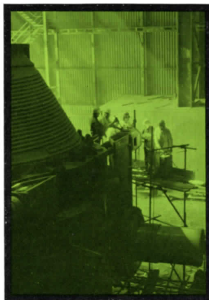
top Prestressing of support tendons on BOS furnace by subcontractor employees above Assembling no2 hood carriage in the charging bay April 1974
