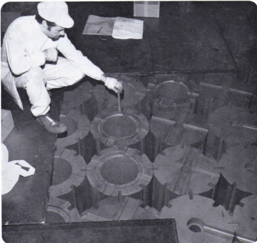
left Hinkley B Ken Lee, Assistant Site Engineer, fits a graphite key into the graphite bricks during the core construction at Hinkley B. Ken is an ex-apprentice from the HW Training School.
